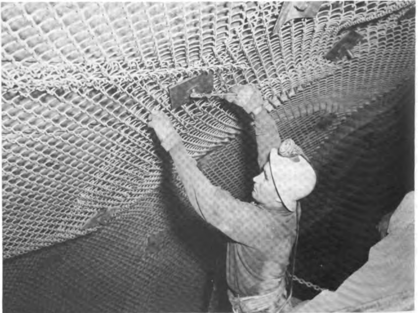
FIGURE 19 Rock bolts and wire mesh reinforce rock to support itself (U.S.A. Corps of Engineers).
